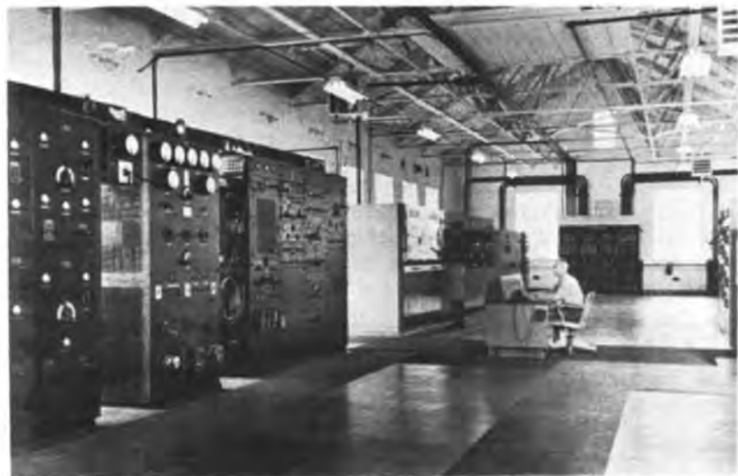
1948 - "WCC" TRANSMITTER SITE, CAPE COD SOUTH CHATHAM, MASS. FRED KREMP - ENGINEER IN CHARGE.
